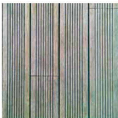
Weathered and dirty floors
