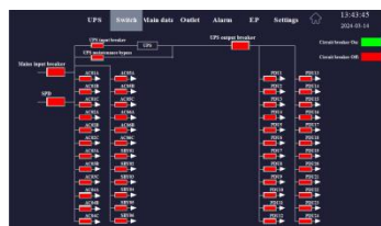
Breaker status monitor
