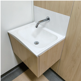
Recessed Bathroom Fixtures
