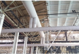
Fabric Air Ducts
