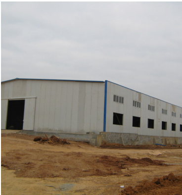
Gabon Plant Project
