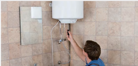
Water heater inlet boosting
